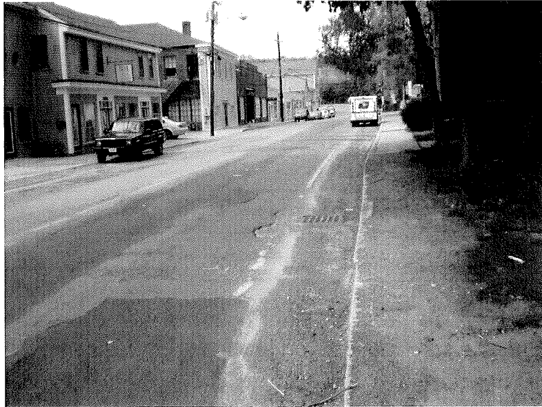
Photo 3 – South Main Street - Poor Road and Sidewalk Condition
