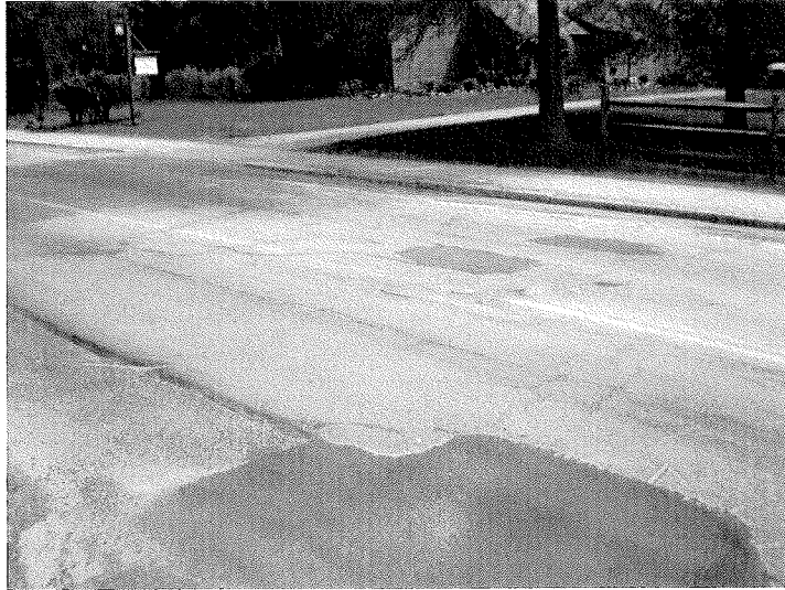
Photo 1 - South Main Street - Poor Road Condition
