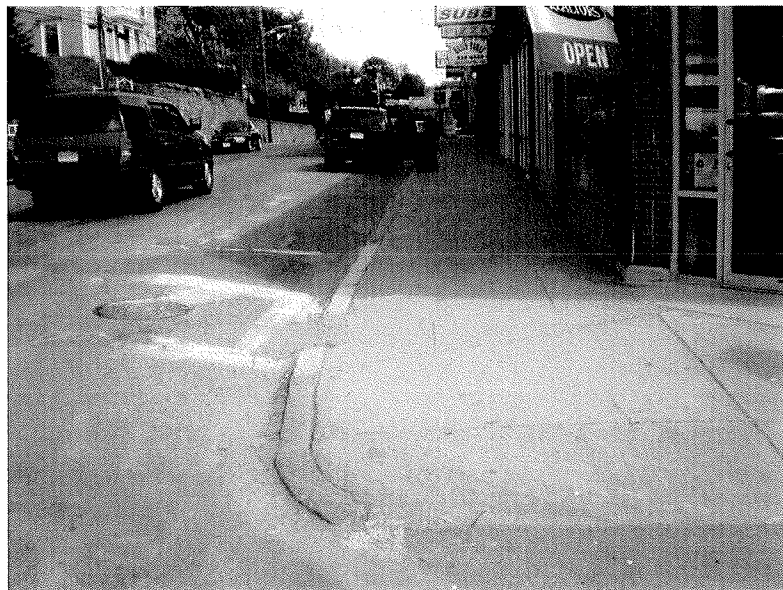
Photo 6 – Central Street - Poor Road and Sidewalk Condition
