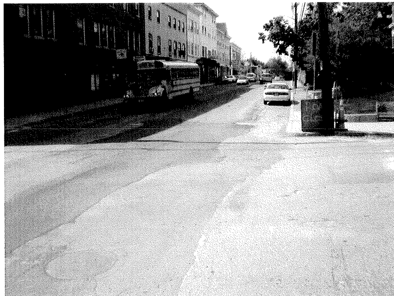
Photo 4 – Central Street - Poor Road Condition
