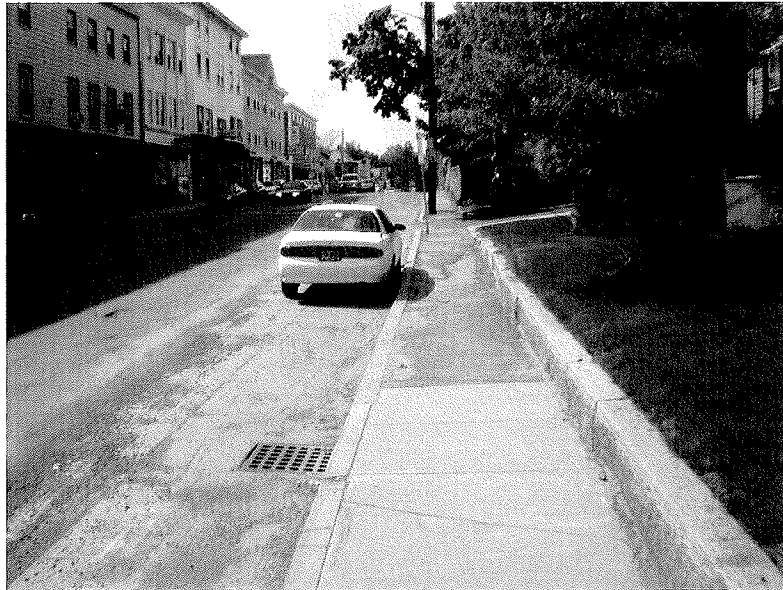
Photo 5 – Central Street - Poor Road and Sidewalk Condition
