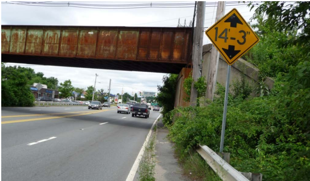
Sidewalk conditions under the Danvers Rail Trail bridge
