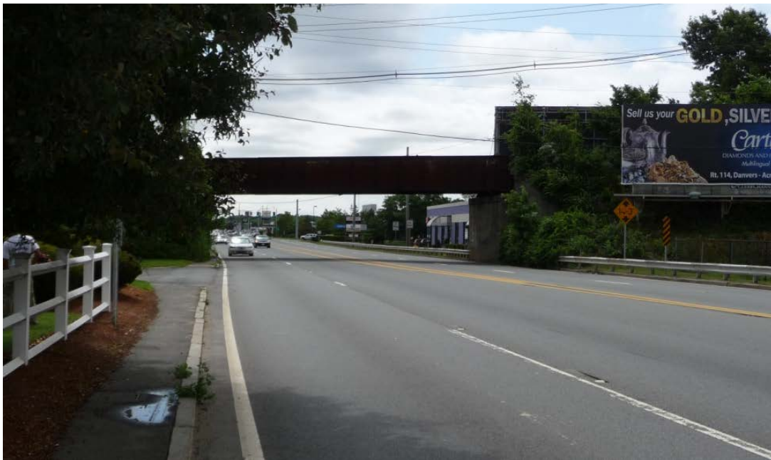
Roadway conditions near the Danvers Rail Trail bridge
